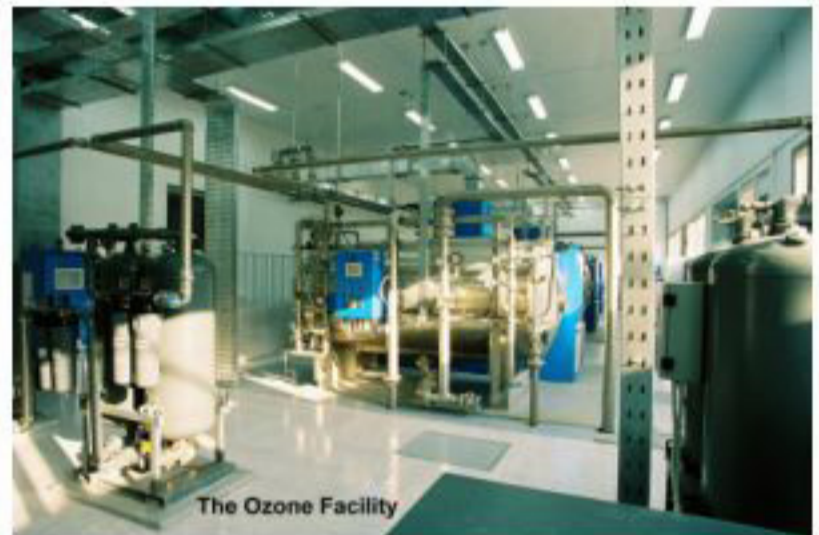
Above – Typical Large-scale municipal drinking water plant
